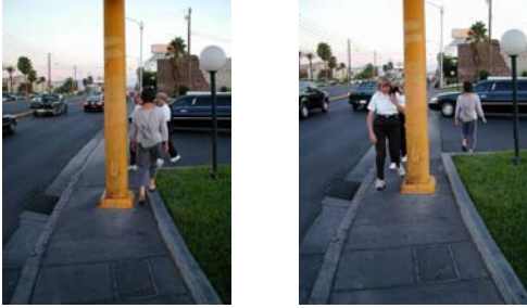
Utilities & poles clutter sidewalk
