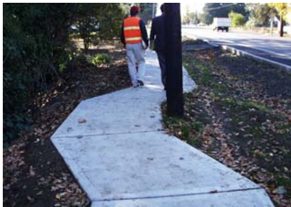
Sidewalk can wrap around pole
