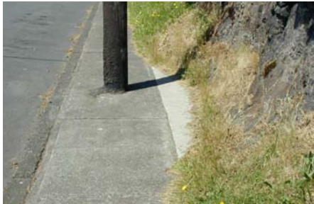
Narrow curbside sidewalk needs mitigation around every obstacle
